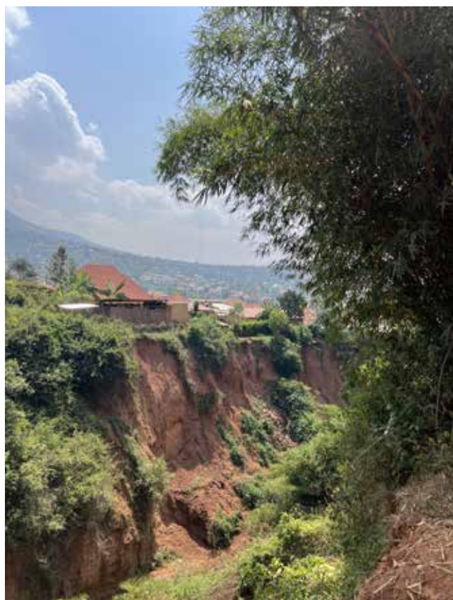
FIGURE 9 | An example demonstrating the common problem of landslides and erosion in the City of Kigali
