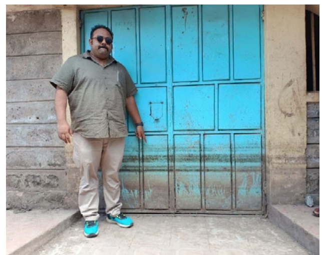
Figure 10 | Flood mark in a house in Mukuru kwa Reuben which is located in a floodplain
